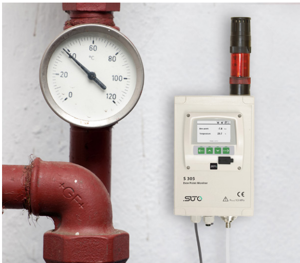
Alarm adjustment at dew point sensor
